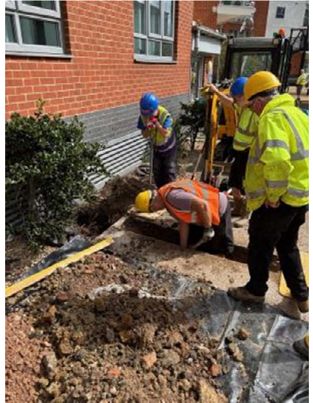
Above and opposite: the work in progress. The completed bollard can be seen in the picture on the back page.
