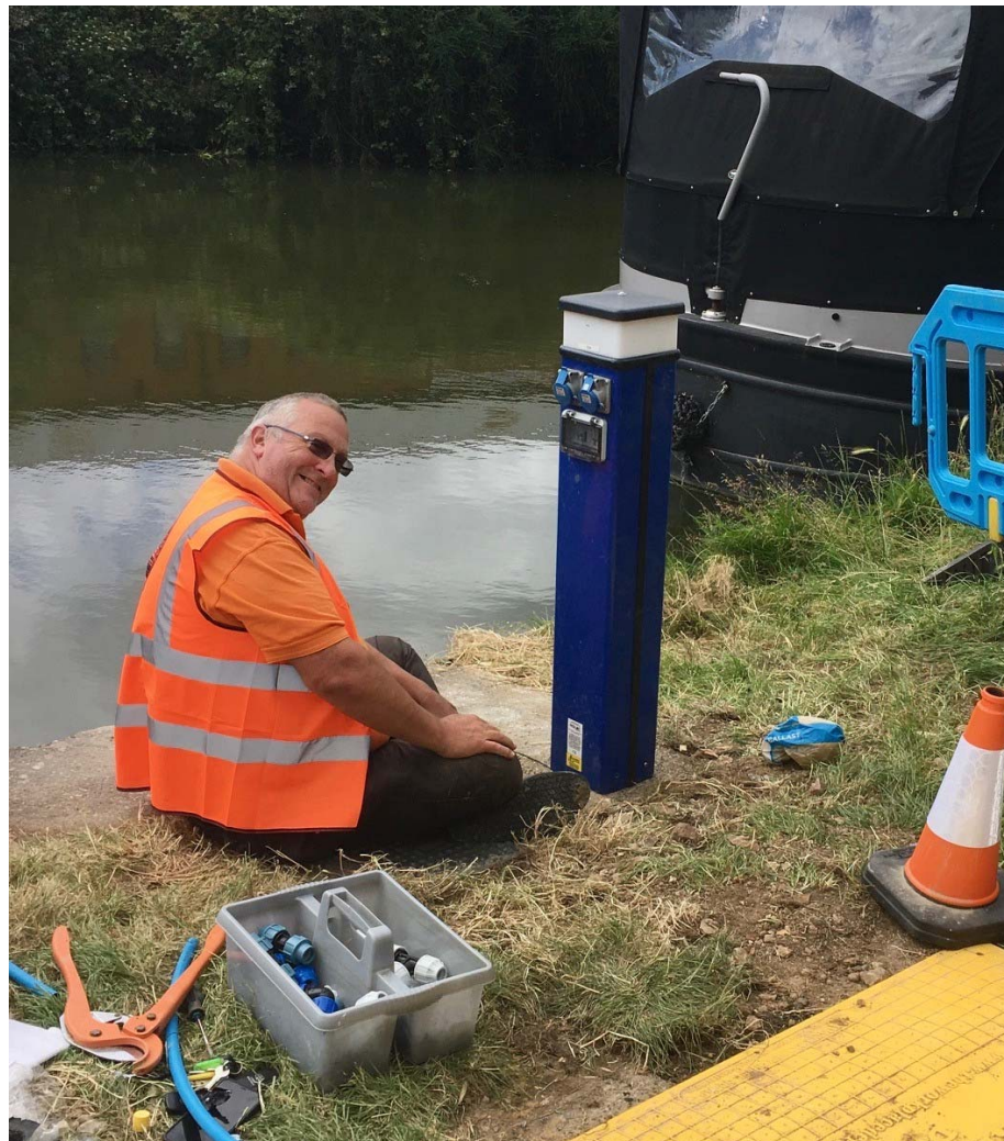
Terry Cavender of Buckingham Canal Limited adding the finishing touches to a smart, blue charging bollard.
